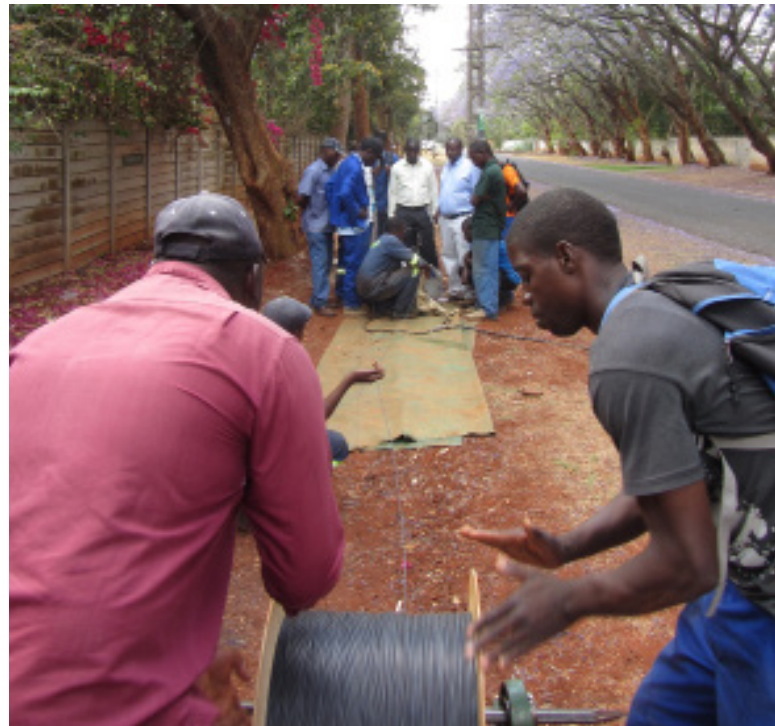
Miniflex® cable being pushed through 5 & 8 mm microduct over distances greater than 150 m
